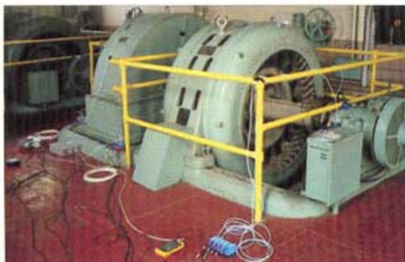
The Pelton wheel (left) and generator (right) instrumented with temporary proximity probes for diagnostic analysis.
