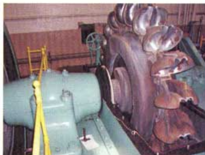
The center pedestal (Bearing 2) in close proximity to the Pelton wheel (right).
